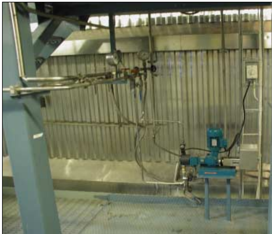
Figure 45. Ammonia feeding equipment
