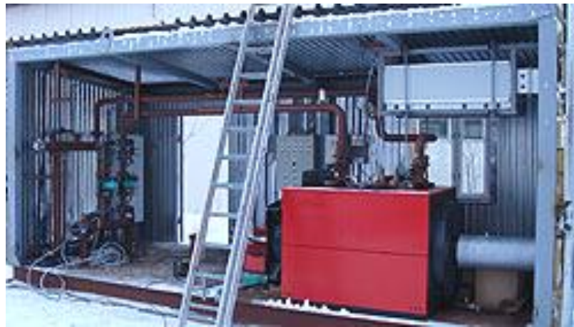
Figure 10. Modular boiler plant
