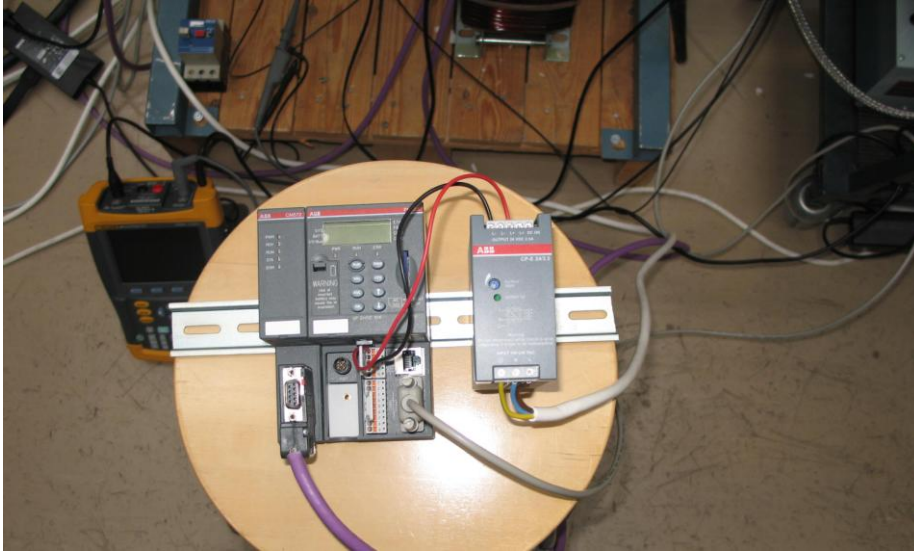
Figure 1.5 ABB AC500 PLC system with Profibus adapter and cable attached to it.
