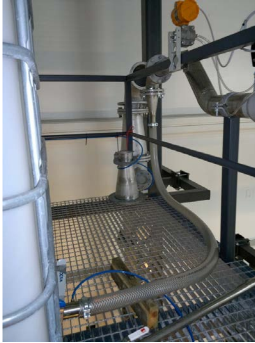
Fig. 4.2 View next to the destination reservoir. The flexible tube increases the flow losses in the system and chokes the liquid supply.
