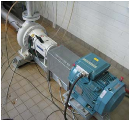
Fig. 2. Sulzer laboratory pumping system that comprises a Sulzer APP22-80 centrifugal pump, an 11 kW ABB induction motor, and an ABB ACS 800 variable speed drive.
