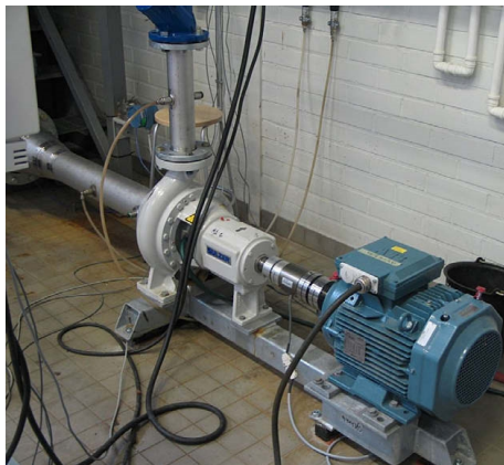
Figure 3.12. Pump drive attached to the piping system. The pump drive consists of a centrifugal pump, an 11 kW induction motor, and an industrial drive.
