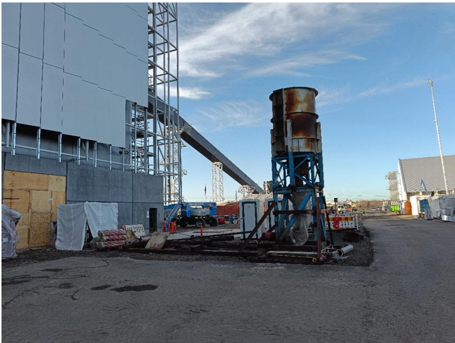
Figure 7. Steam blowing silencer in construction phase (Valteri Liimatainen).
