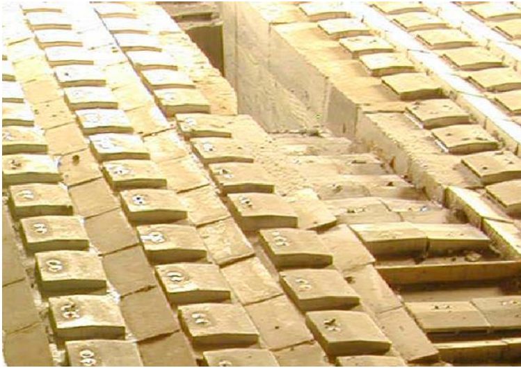
Figure 11. Step grate of a BFB boiler (Sumitomo SHI FW 2024).
